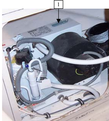
AIR CONDITIONING SYSTEM IN V-BERTH
