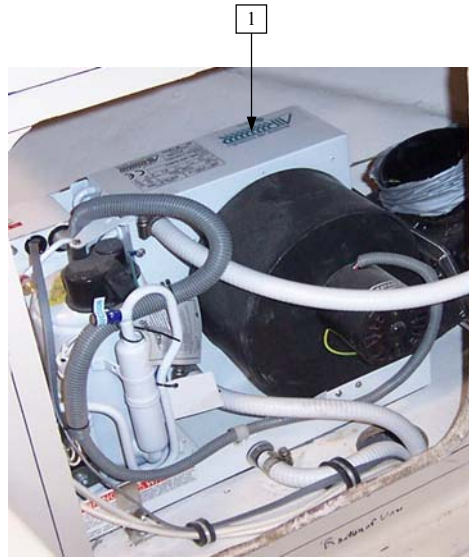
AIR CONDITIONING SYSTEM IN V-BERTH
