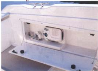
Air Compressor & Transom Shower
