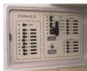
AC/DC Distribution Panel
