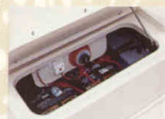
Typical pre-rigged electrical and fuel system installation.
